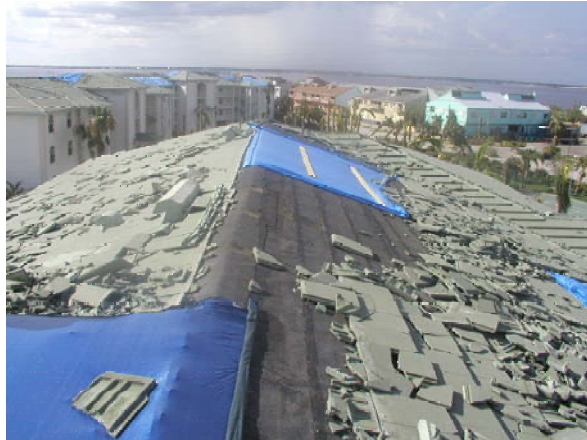
Example of a ridge tile failure in a concrete tile roof system. Photo courtesy of Mr. Warren French of French Engineering, Inc.
