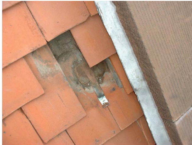
Clay overlapping (flat shingle) tile exhibiting signs of water absorption. Photo courtesy of the author.
