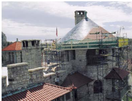
Process of replacing original Ludowici Celadon clay Spanish tile (initially installed at the turn of the 20 th century) with new tile by the same manufacturer on a historic hotel in upstate New York (the original tile came from Celadon’s plant in Alfred, NY).
