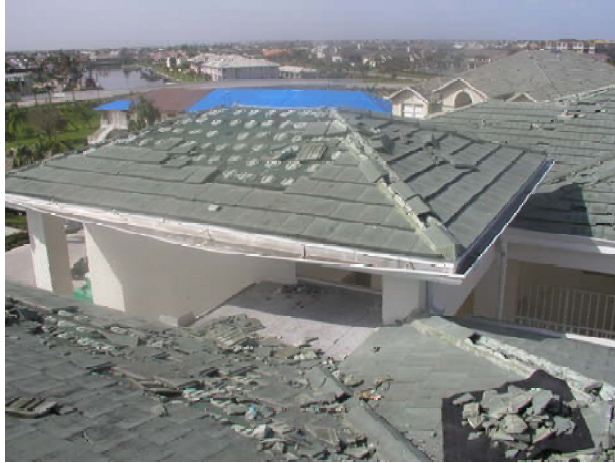
Upper concrete tile roof exhibiting partial failure of the “foam set” system possibly due to an improper foam mix. Lower roof exhibiting damage from flying debris. Photo courtesy of Mr. Warren French of French Engineering, Inc.
